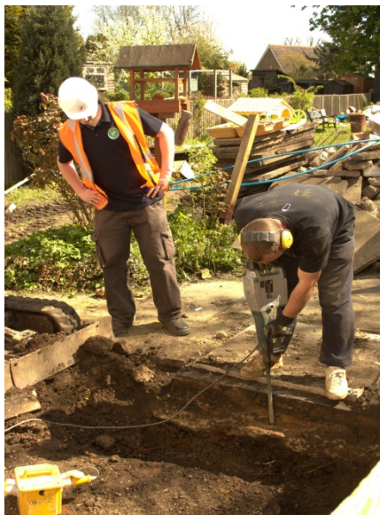
DP5: Shot of Victorian toilet block and brick work, during removal, facing SE.
