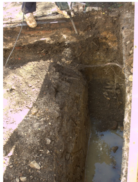
DP6: Victorian toilet block and brick work and foundation trench, facing SE.
