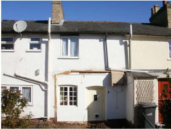
DP3: Shot of Rear of Property, notice scar of removed lean-to, facing NW.
